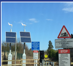
Wind & Solar Powered Rail Crossing
